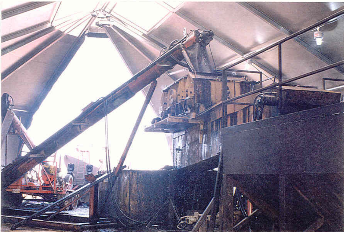
Figure 4. Site B injection equipment in operation. Enclosed SFI equipment at this site allows year-round operations during inclement weather.
