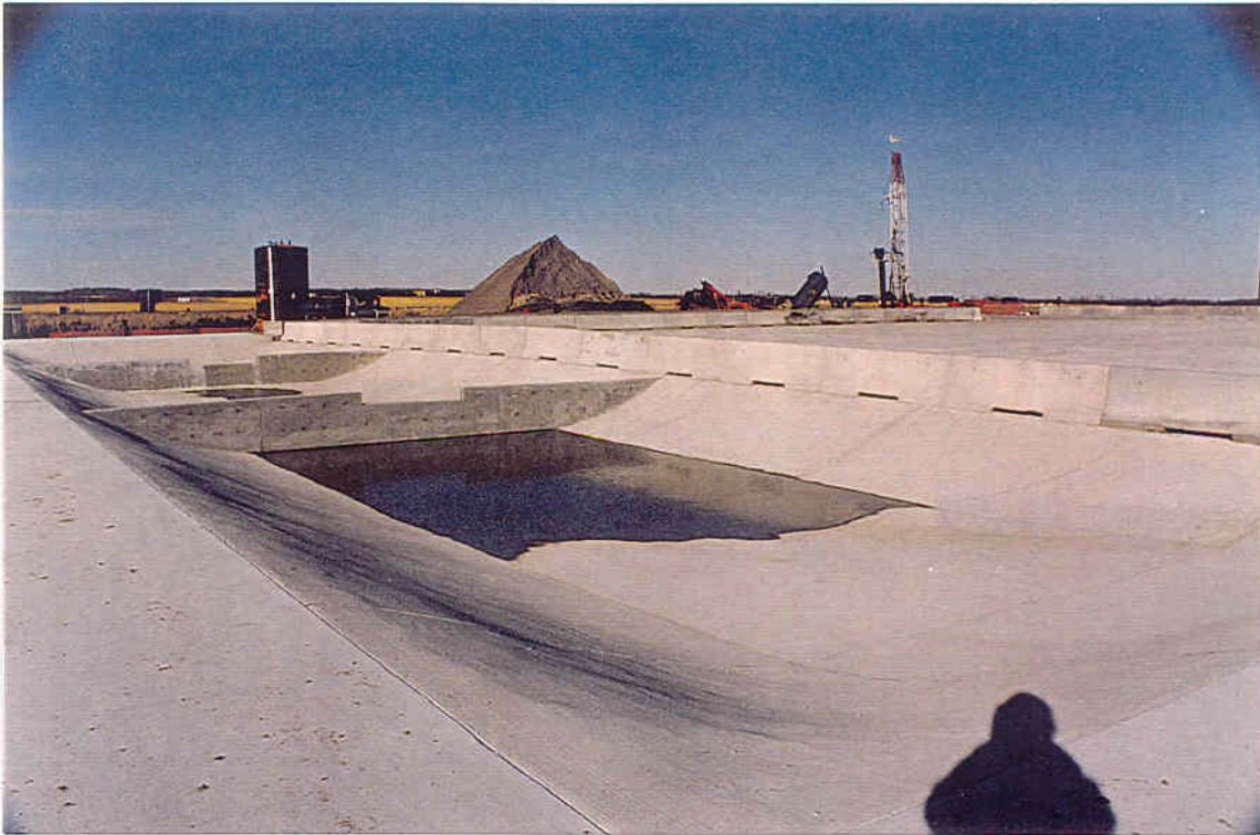
Figure 3. Site A surface layout. Produced sand stockpile to be injected is visible in background between water tank and well, which is being worked over. In foreground is new concrete and clay lined waste storage pit .
